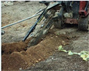
A trencher attachment digs the ditch for an electrical line as well as a drainage trough for the fire pit.
