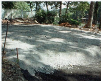
The bed of crushed rock should be spread evenly over the patio site and thoroughly compacted.
