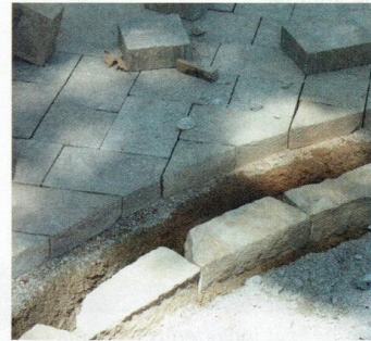
The fire pit was surrounded by the circular edge of the patio, which had to be cut at an arc.
