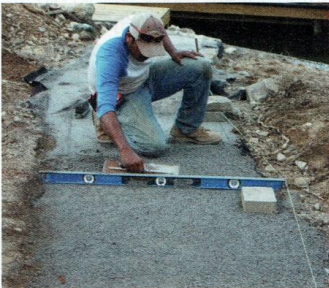
The grade of the site sloped significantly in different directions along the the walking path.
