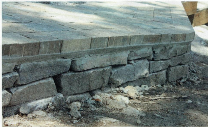
To accommodate the slope, a drystack stone wall was built to support the downhill side of the walkway, and the edge pavers were mortared onto the wall as the top course.
