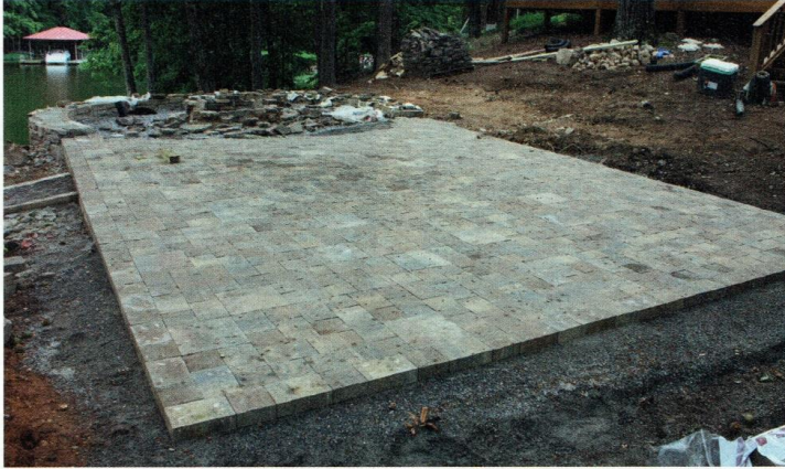
The exposed edges of the pavers will be buried by substantial landscaping so the patio surface will be just above ground level.
