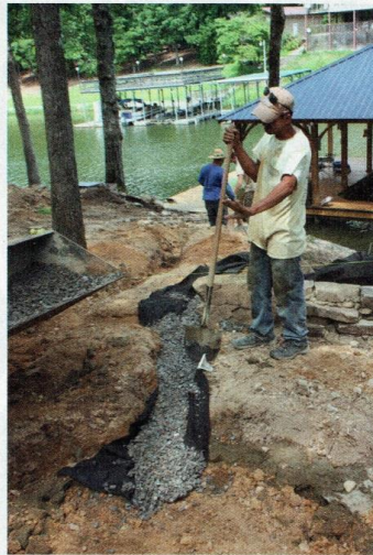
Site conditions and patio design will determine how to manage drainage. This patio included a circular fire pit with a drainage trench, which was lined with landscape fabric and filled with gravel.
