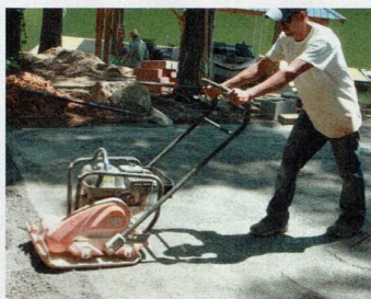
A vibratory plate compactor will be used in multiple phases of construction.
