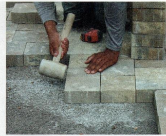
A rubber mallet should be used to set the pavers into the base.
