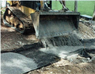
The project included three walking paths, which were constructed much like the patio.
