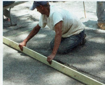
The bed of crushed rock should be screeded evenly in preparation for the paver surface.
