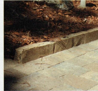
The uphill side of the patio was lined with tall edging bricks to divert runoff from the patio surface.
