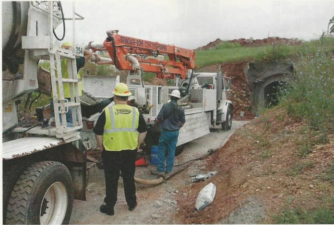
Fig. 6: Schwing S17 with 180-degree discharge serves as line pump for shotcreting up to 400 ft (120 m) inside the tunnel
