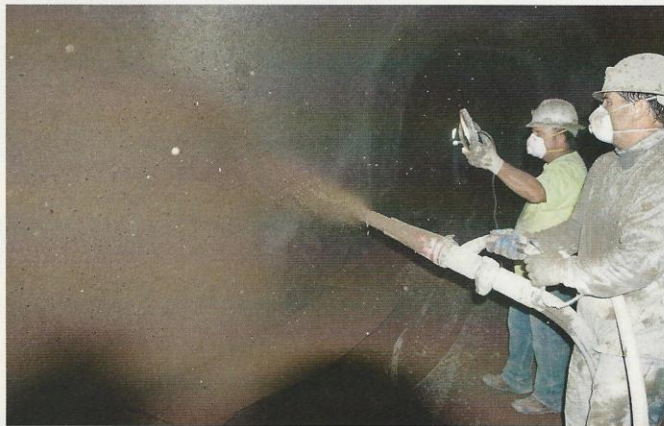
Fig. 4: Wet-mix shotcrete was applied 6 in. (150 mm) thick over welded wire reinforcement in four passes
