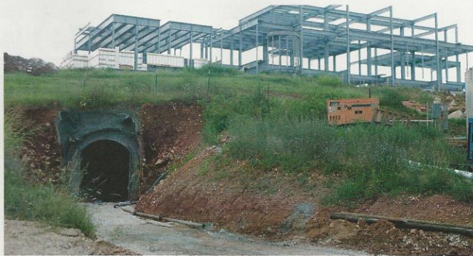
Fig. 3: Exterior portal leads to 150 ft (45 m) long tunnel and various chambers to create a wine cave 45 ft (14 m) under the owner's new home
