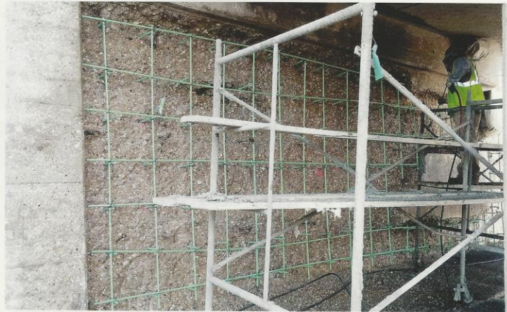
Fig. 1: Repair areas were found to be not only much larger in the field but also deeper than was called out on the plans and also lacking any reinforcing bar
