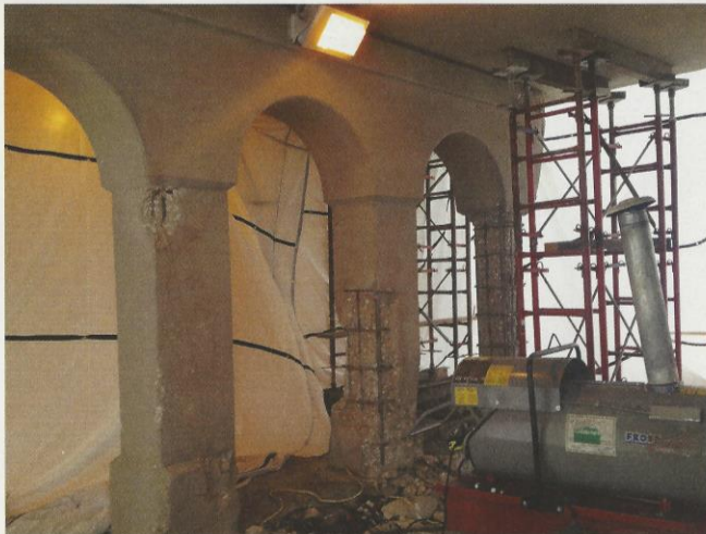
Fig. 5: Large propane heaters kept temperatures inside enclosure within specifications during cold winter months
