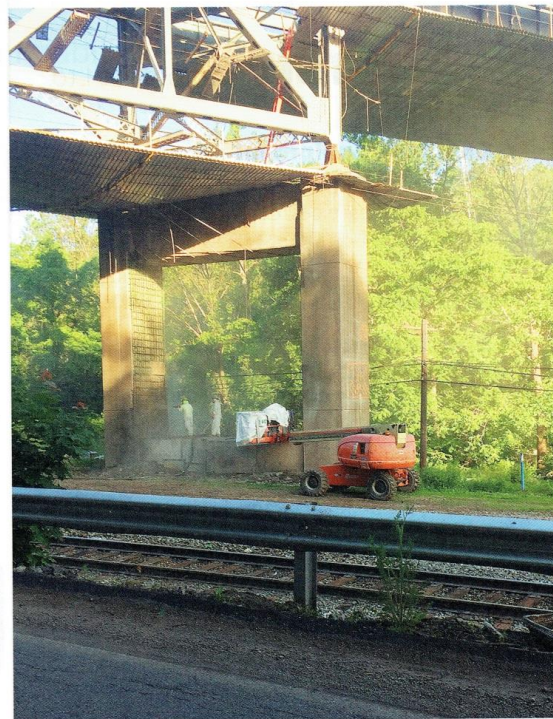
Material being pre-dampened and gunned onto a cap beam on a bridge in West Mifflin, PA
